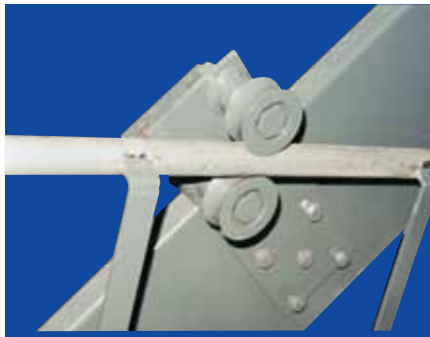
Handrail Roller Guides
